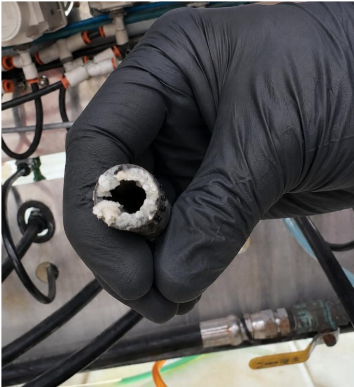
Figure 1 - 1/2" Polyline Detergent Buildup
