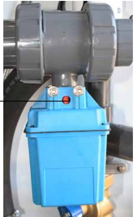
View Port on Recirc Valve: Green for open
